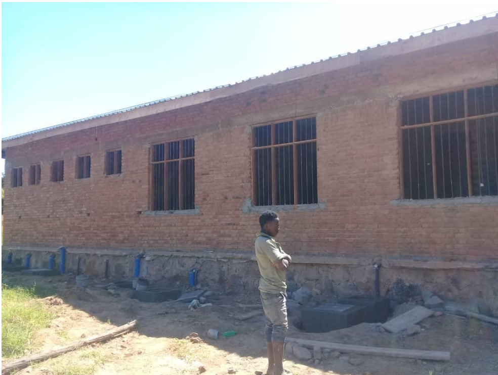
Photo taken in June 2018: Window frames and waste water pipes (two lines) with cleaning boxes
